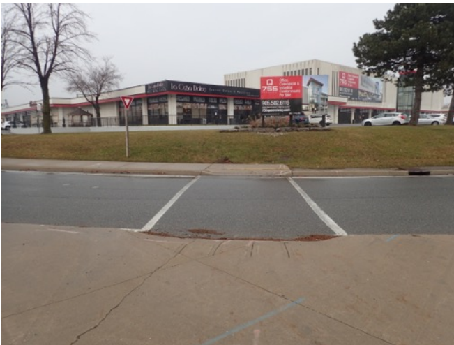
Image 7: View of paved roadway, pedestrian sidewalk, traffic island and low embankment at the northeast corner of the Cawthra Road-Queensway East intersection.
