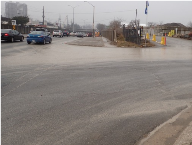
Image 9: View of paved roadway, sidewalk and retaining wall along Cawthra Road north of Needham Lane.
