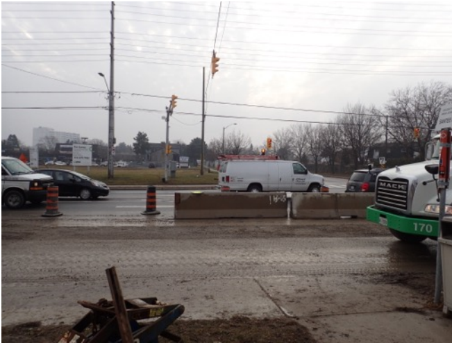
Image 13: View of paved roadway, sidewalks, utility installations, grassed margins and active worksite at intersection of Cawthra Road and Silver Creek Boulevard
