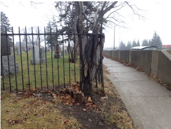
Image 31: View of retaining wall, paved sidewalk and grass strip at the west margin of Dixie Union Cemetery.
