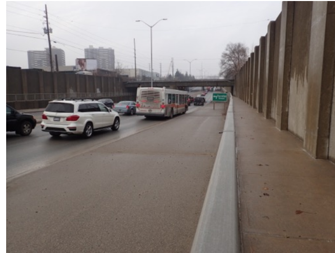
Image 10: View of paved roadway, pedestrian sidewalk and retaining walls along, and railroad bridge structure over, Cawthra Road.
