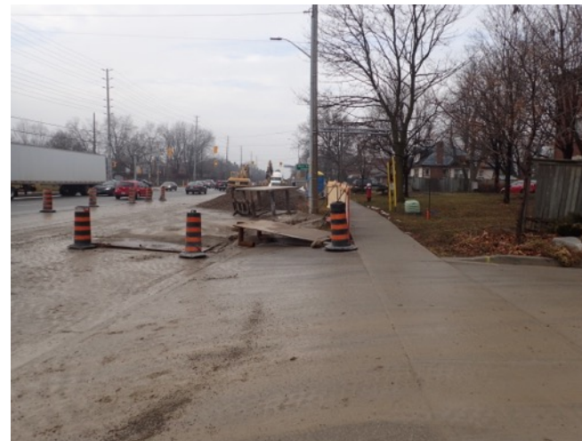
Image 12: View of paved roadway, sidewalk, utility installations, graded margins and active worksite along the east side of Cawthra Road opposite Silver Creek Boulevard.
