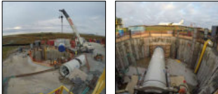
Shaft site for the twinning of the Etobicoke Creek Sanitary Trunk Sewer under Runway 23 at Lester B. Pearson International Airport
