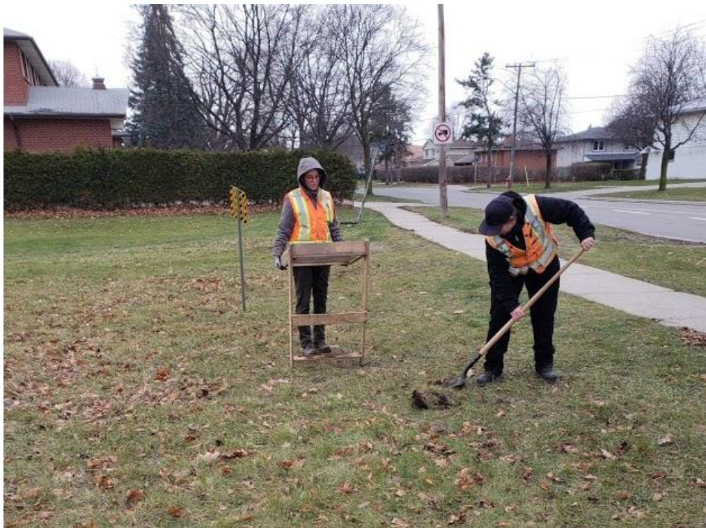
Image 12: Test pit survey in progress at preferred shaft location 09C, facing north, 27 November 2020.
