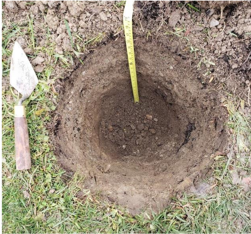
Image 23: Example of test pit at preferred shaft location 17C exhibiting disturbance, facing north, 26 November 2020.
