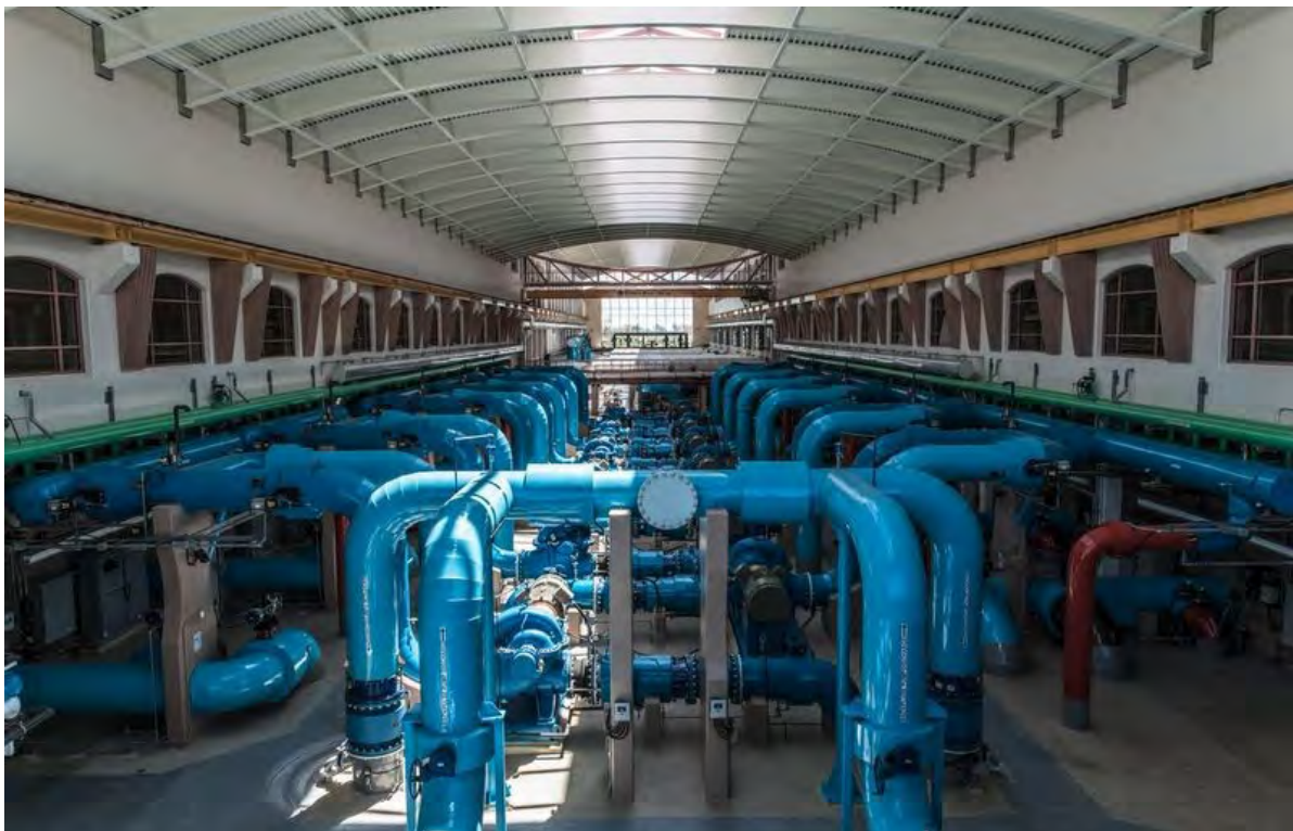
Figure 3: The pumps and pipes of a membrane water treatment system at the Lakeview Water Treatment Plant.
