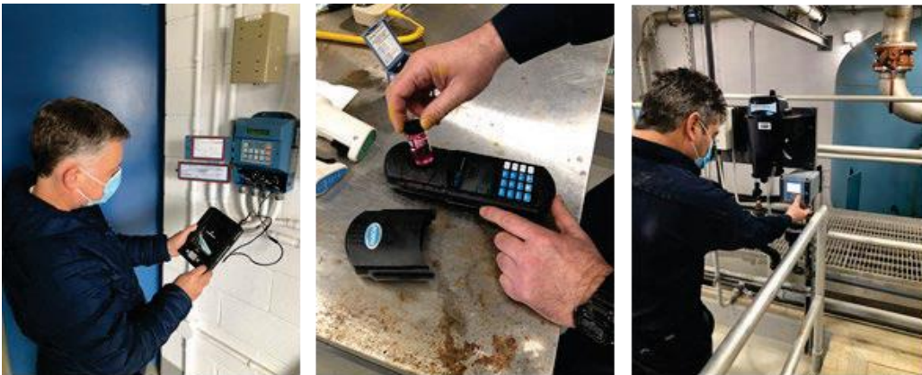
Figure 10. Staff calibrating level transmitter and verifying handheld chlorine analyzer and online turbidity analyzer
