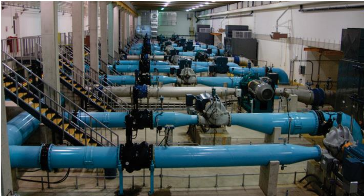
Figure 2. Airport Road Reservoir and Pumping Station, pump room
