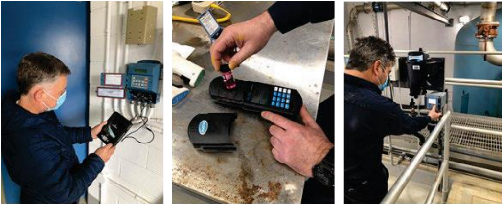
Figure 14. Staff calibrating level transmitter and verifying handheld chlorine analyzer and online turbidity analyzer
