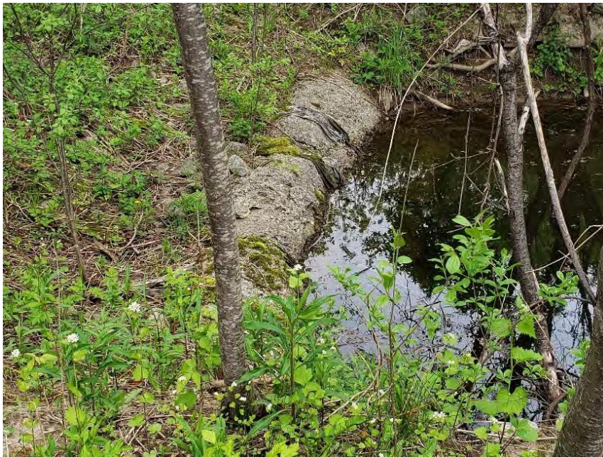
Figure 1-5. Eroded Ground Cover and Adjacent Pit
