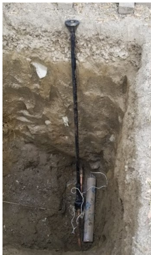
Copper water service with valve and anode to prevent corrosion.
