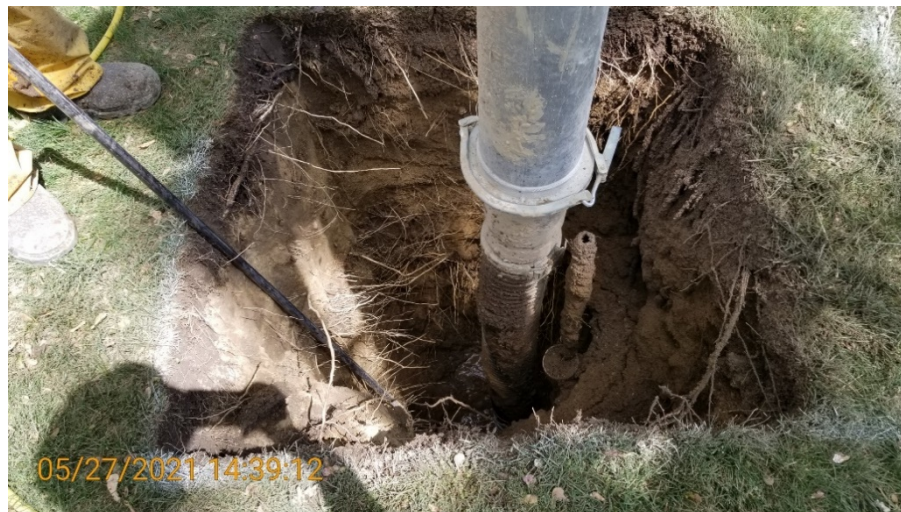
Hydro vacuum excavation uses water and vacuum technology to safely excavate around more sensitive areas.
