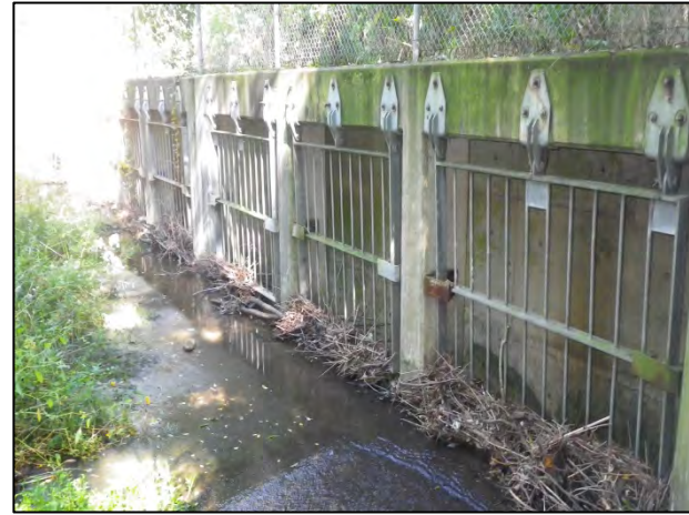
Tributary 2 of Mullet Creek: Overlooking pipe inlet approximately 30 m west of Derry Road.
