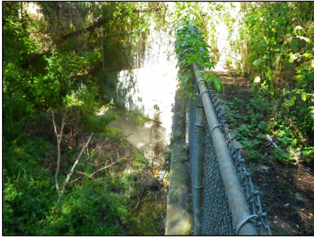
Tributary 2 of Mullet Creek: Overlooking pipe inlet approximately 30 m west of Derry Road.
