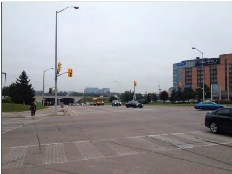
Photo 2-4: Faded Crosswalk Pavement Markings
