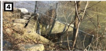
4 Ex. Storm Sewer (Outfall) : maintain and/or remove and replace pipe section during construction.
