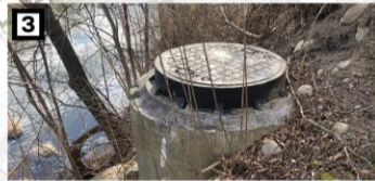
3 Ex. MH adjacent to watercourse and within the bank; determine proper safeguarding of MH sections while not adversely affecting the watercourse and creek bank.
