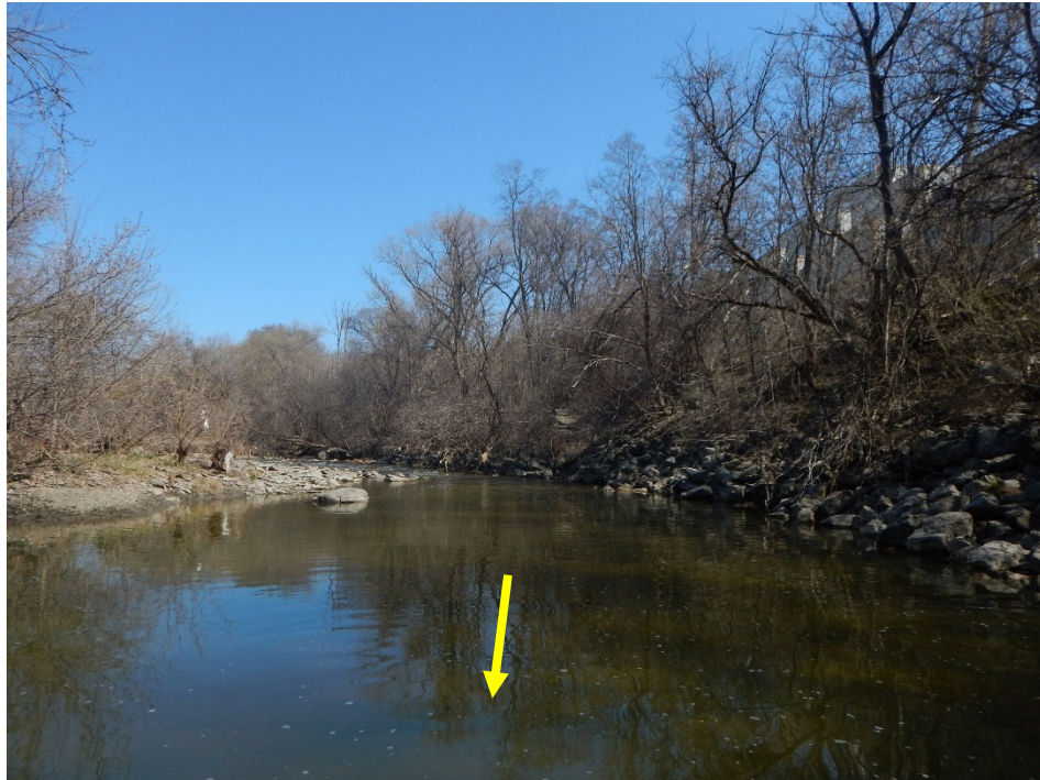
Valley wall contact and existing bank stabilization on left bank through large pool.
