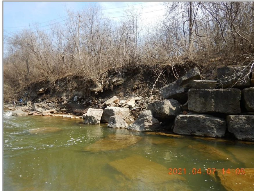
View of failing erosion control measures on the southern channel bank near The West Mall, downstream of the study area.
