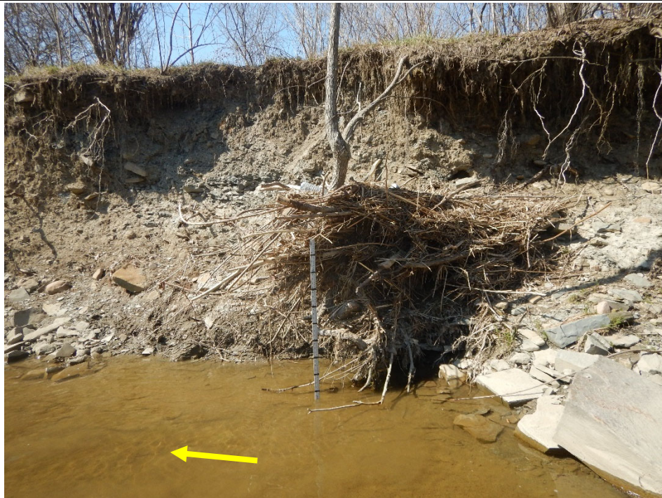
Signs of erosion of right bank downstream of manhole and storm sewer outfall. Note position of trash line.
