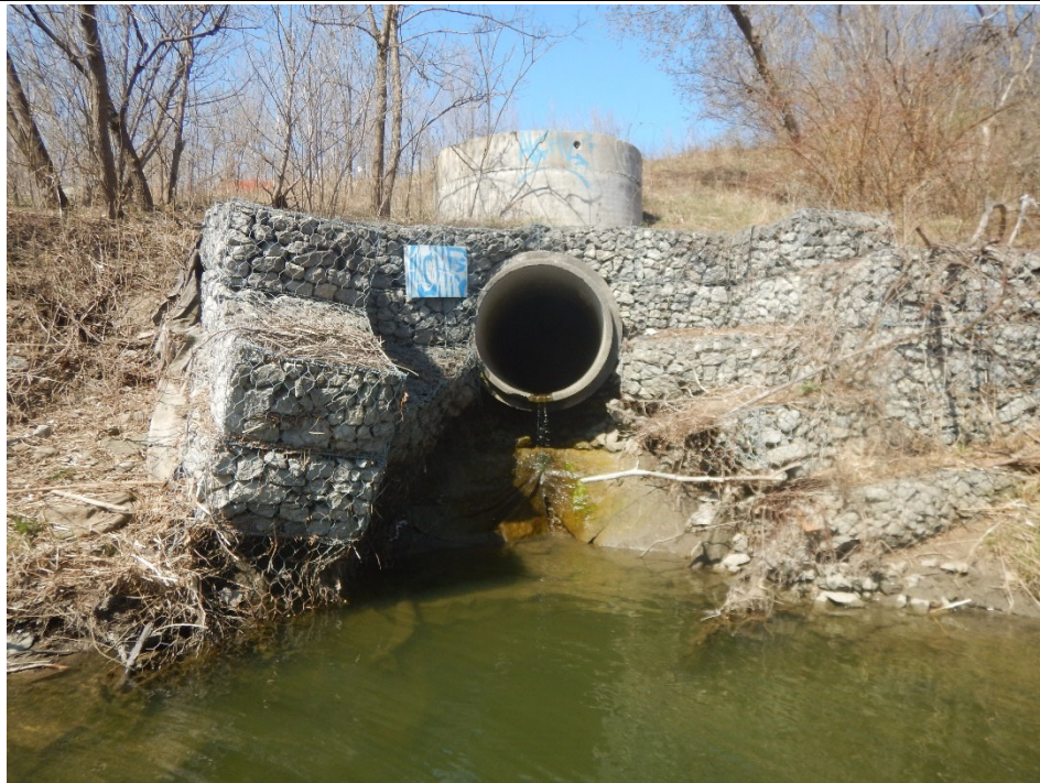
Elevated storm sewer outfall, undermined gabion baskets, and large scour pool south of Southcreek Road.
