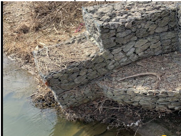
Photo 9: undermined gabion (April 6, 2021).
