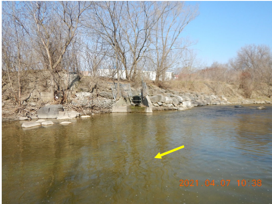
Photo of ETSS manhole, storm sewer outfall, and bank stabilization works installed in 2002.
