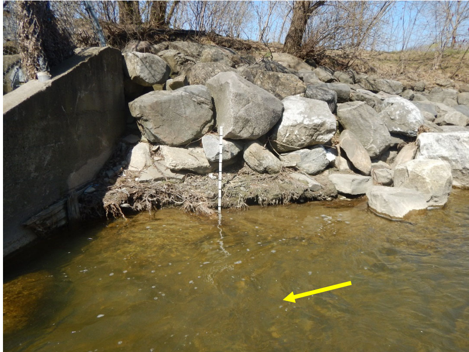
Photo showing erosion control measures installed to protect the storm sewer and ETSS manhole in 2002.
