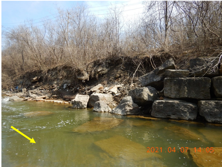
Failing erosion control measures on the left bank downstream of the study area near The West Mall (yellow arrow denotes flow direction).
