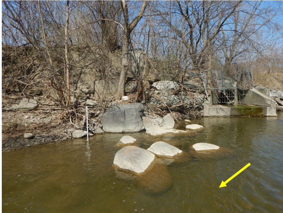
Photo of manhole, storm sewer outfall, and bank stabilization works. Storm sewer is slightly elevated above the channel bed.
