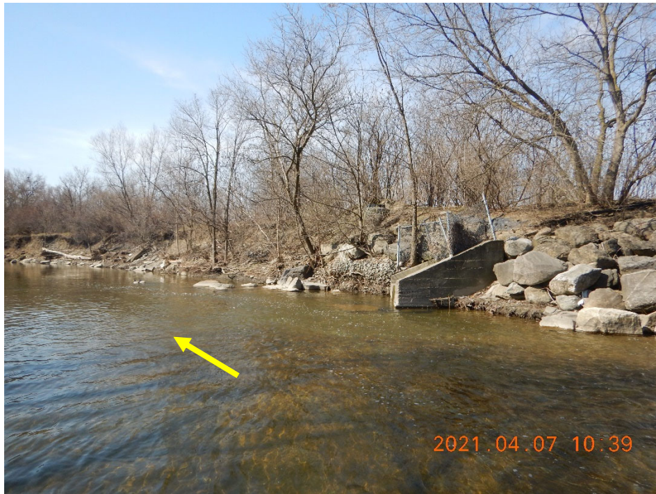
Photo facing right bank showing erosion downstream. Channel has downcut into shale bedrock in vicinity of the ETSS manhole and storm sewer outfall.
