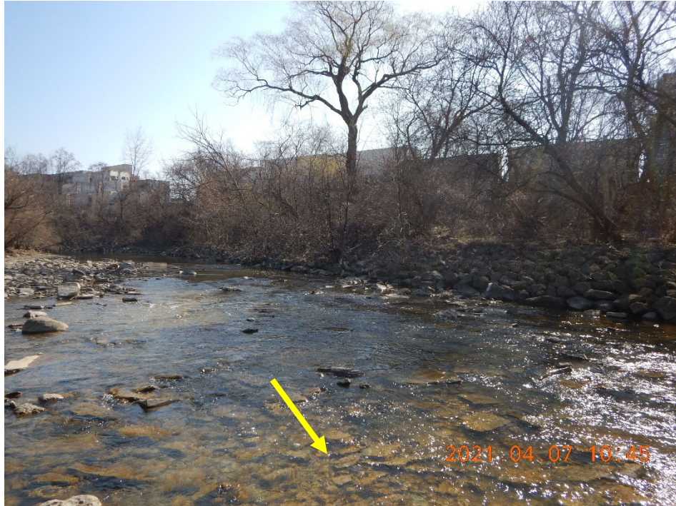
Photo of existing erosion control measures along the left bank upstream of the ETSS manhole and storm sewer outfall.
