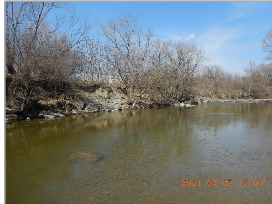
Upstream view towards the MH and storm sewer outfall. Erosion was observed downstream of MH along the western channel bank.
