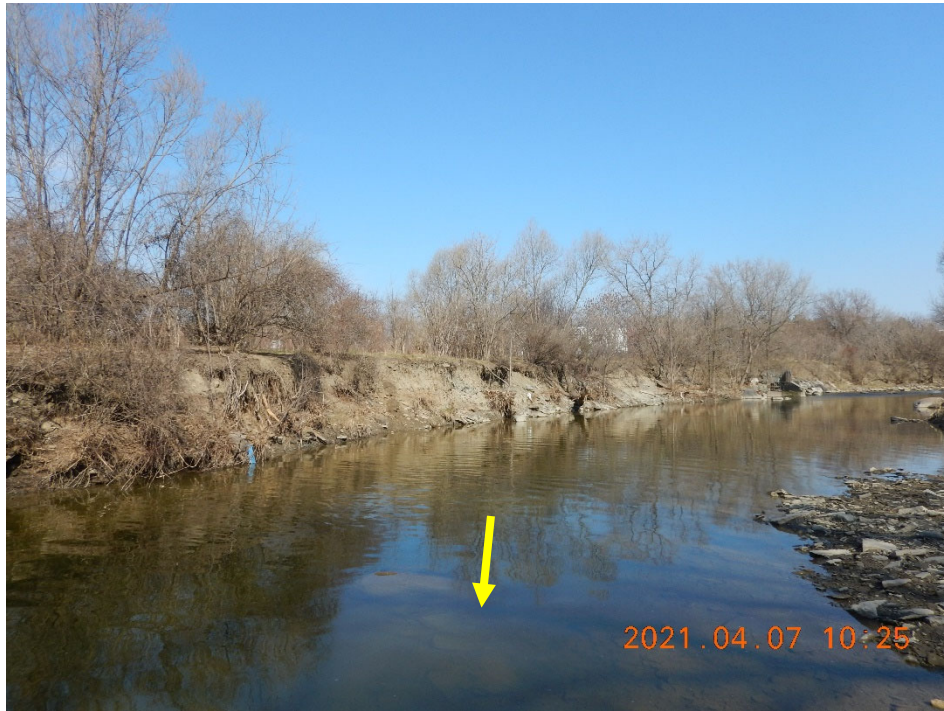
Photo facing upstream towards storm sewer outfall and ETSS manhole. Note extensive erosion on right bank.
