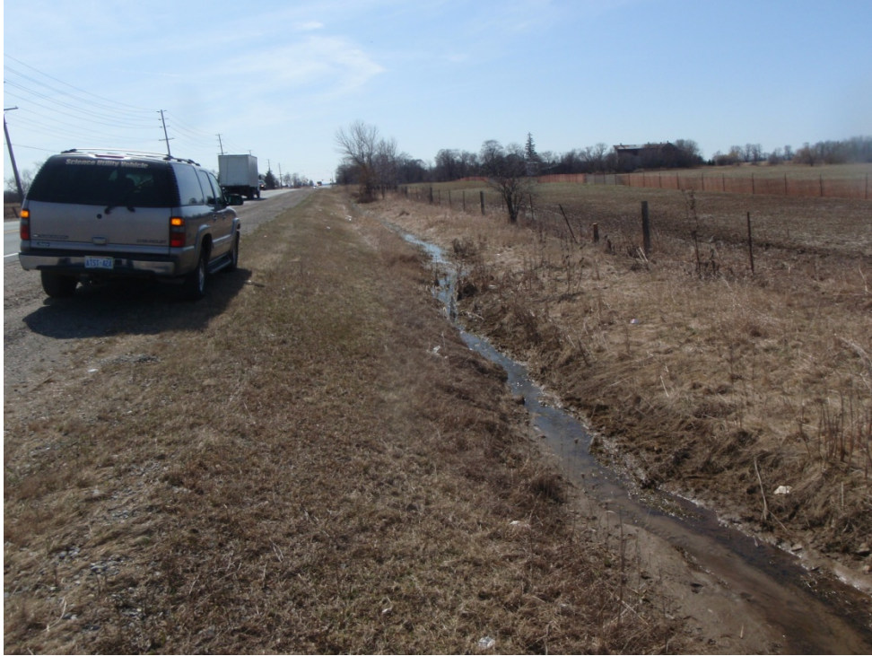
Photograph 11. Ditch flowing easterly to watercourse 3b on upstream side of Bovaird Drive. March 30, 2010.
