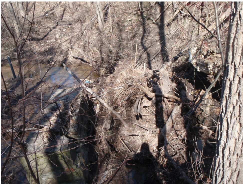
Photograph 2. Debris jam at upstream end of culvert at watercourse 2a. March 30, 2010.
