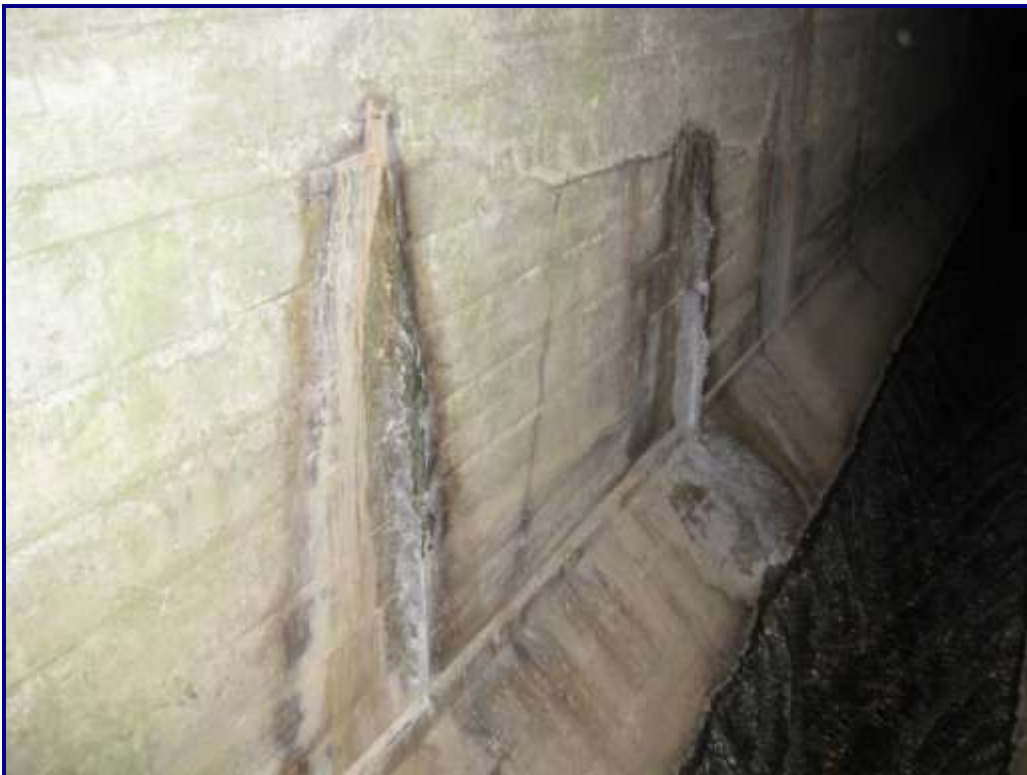
Photo 60 – Structure No. 14: Typical Culvert Wall Cracks
