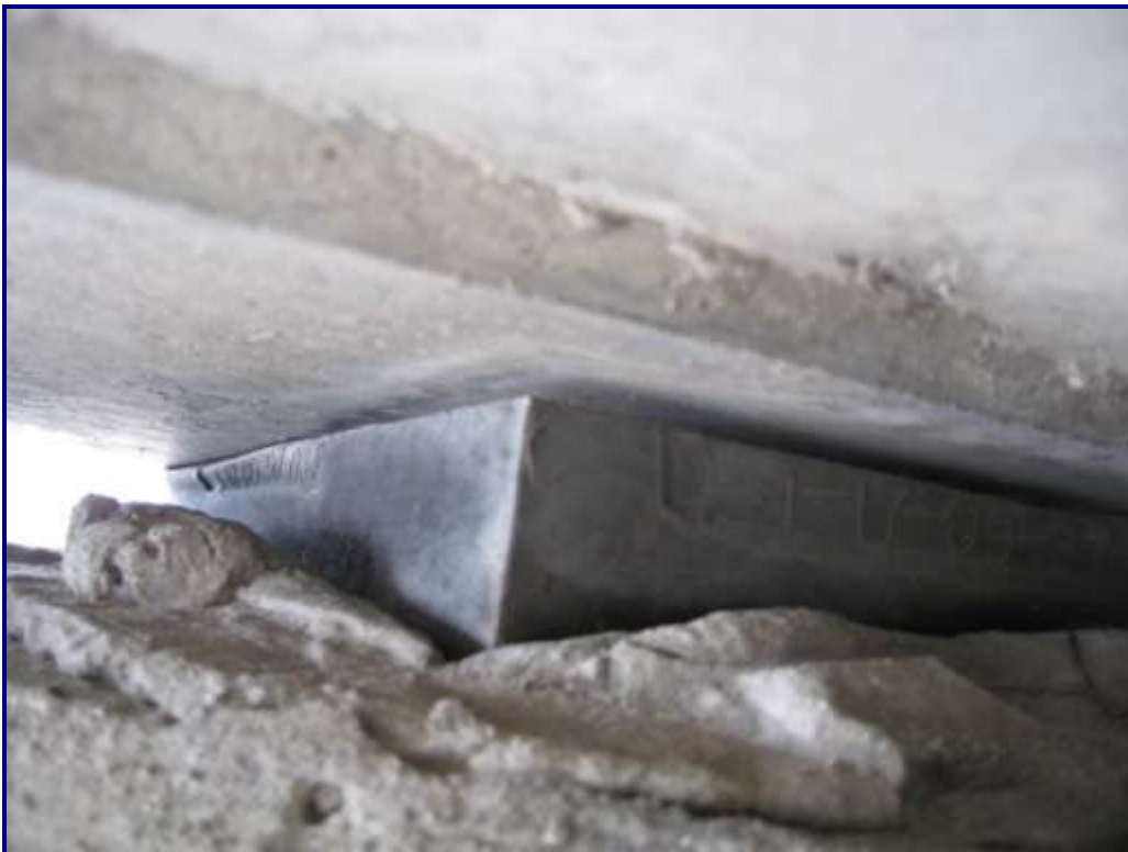
Photo 9 –Structure No. 2: Light Cracking on Bearings – Gap between Girder and T/Bearing Pad
