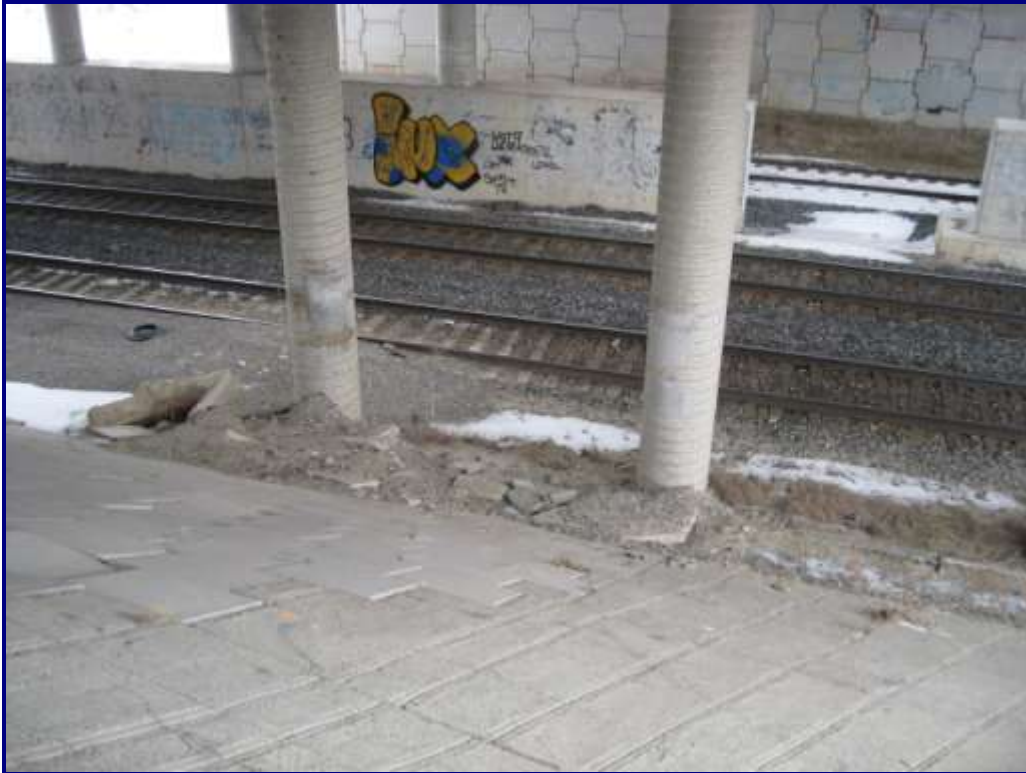
Photo 6 – Structure No. 2: Two Tracks – Centre Span 1 Track – West Span Slope Protection Deterioration
