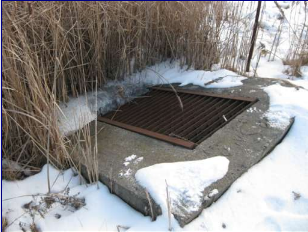
Photo 61 – Structure No.14: Metal Grate Inlet Midway Through Culvert
