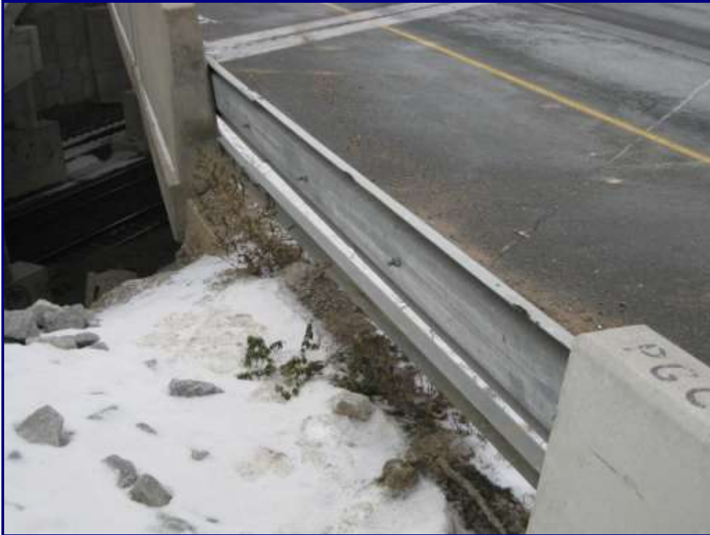
Photo 14 – Structure No. 2: SBGR Posts Missing
