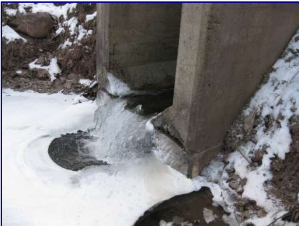
Photo 58 – Structure No.14: Scour Potential at Culvert Outlet
