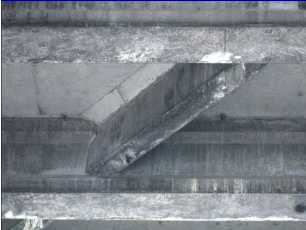
Photo 10 – Structure No. 2: Deterioration of Diaphragm
