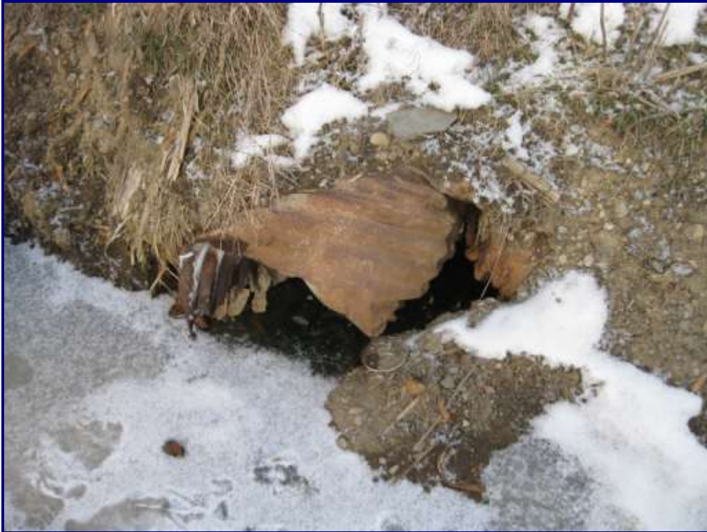
Photo 29 – Structure No. 7: Damaged Culvert End
