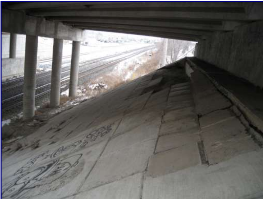
Photo 11 – Structure No. 2: Slope Protection-Footing Exposed
