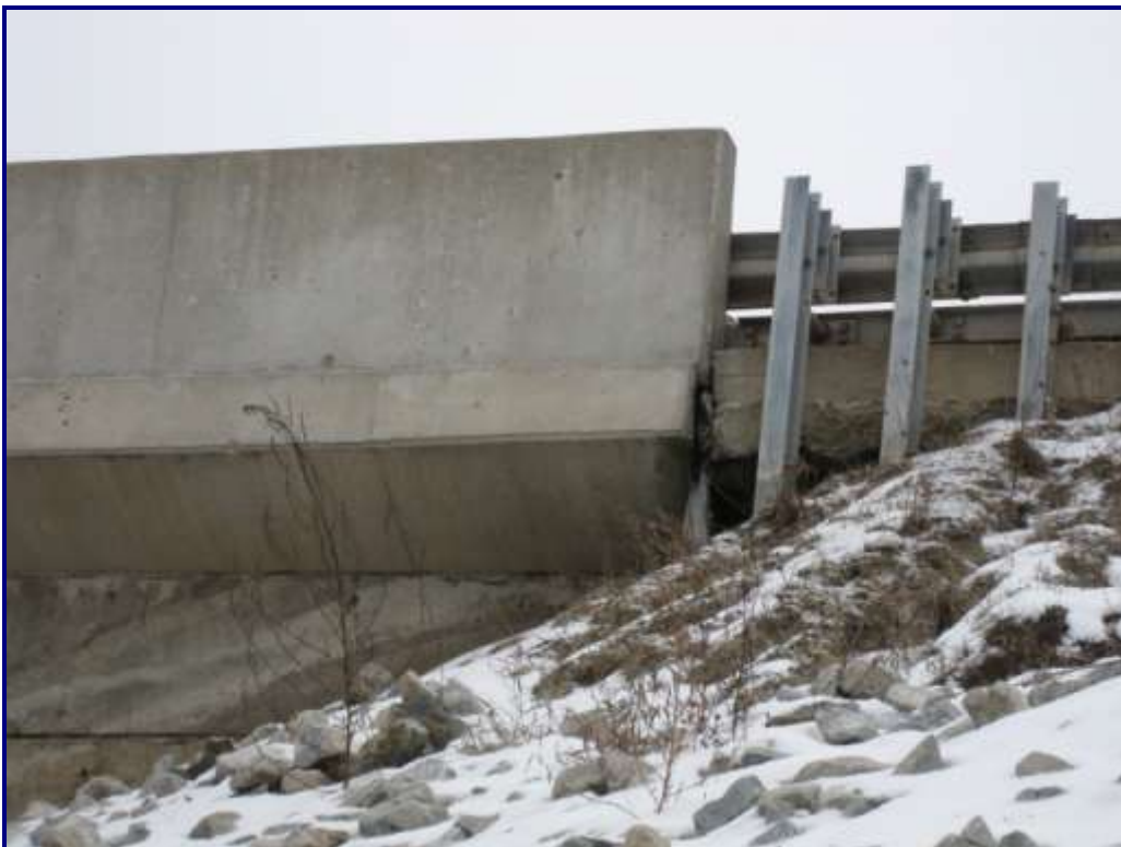
Photo 15 – Structure No. 2: Erosion at End of West Wingwall – North Side
