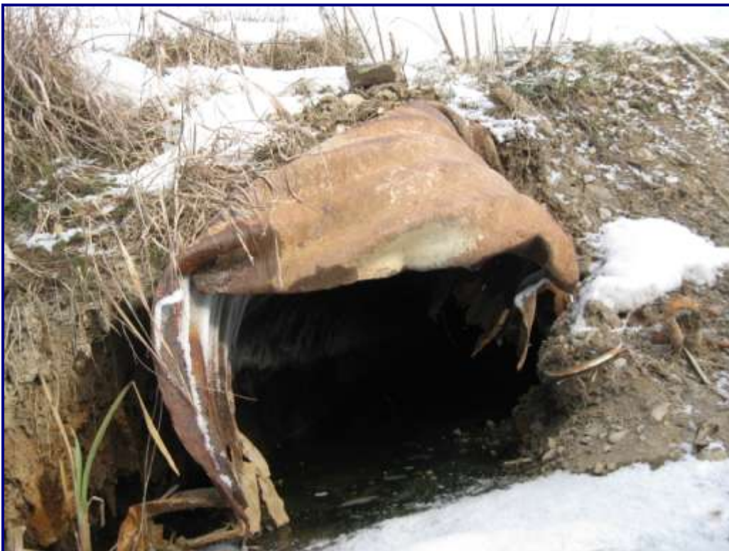
Photo 30 – Structure No. 7: Damaged Culvert End
