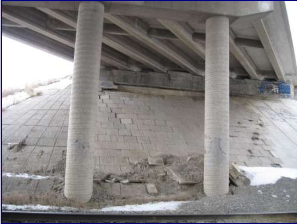
Photo 12 – Structure No. 2: Protection Deterioration
