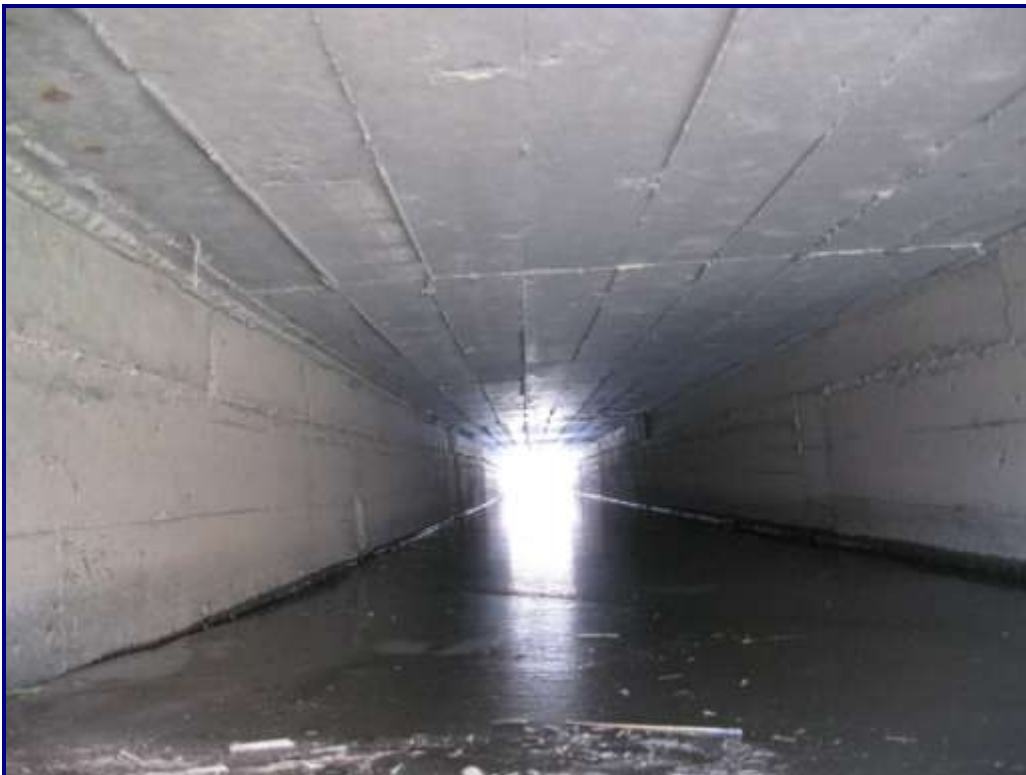
Photo 42 – Structure No. 10: South Barrel Looking North
