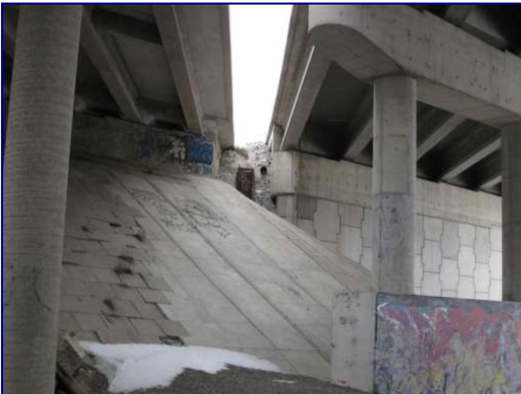
Photo 13 – Structure No. 2: Slope Protection Deterioration and RSS Wall
