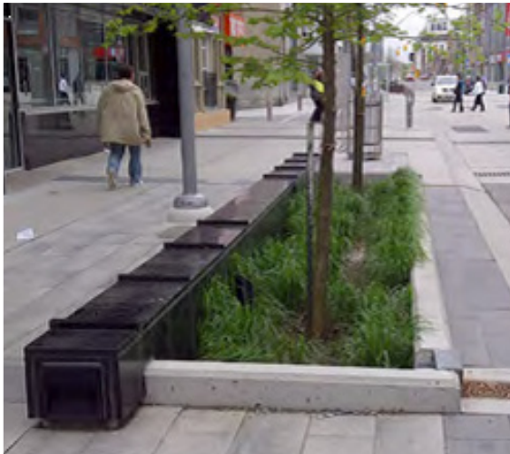
Bioretention planter (Source: CVC)
