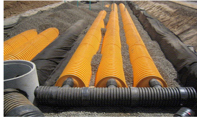
Infiltration Chamber (Source: Region of Peel)
