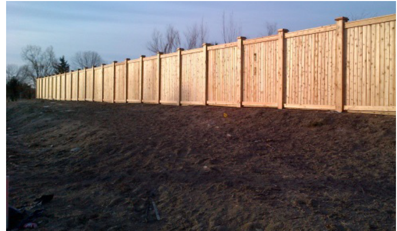
Wooden Noise Attenuation Wall (Source: Region of Peel)
