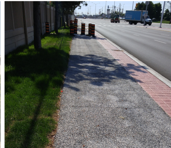
Pervious Concrete Sidewalk (Source: Region of Peel)
