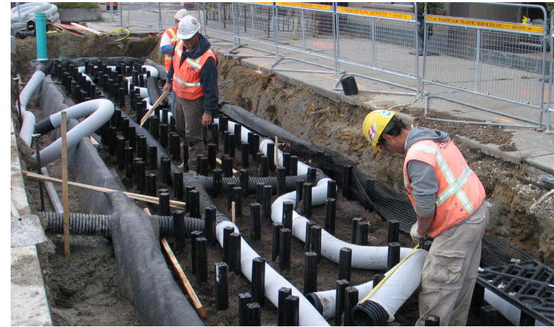
Soil support system being installed under a sidewalk in Toronto (Source: Deep Root Inc.)
